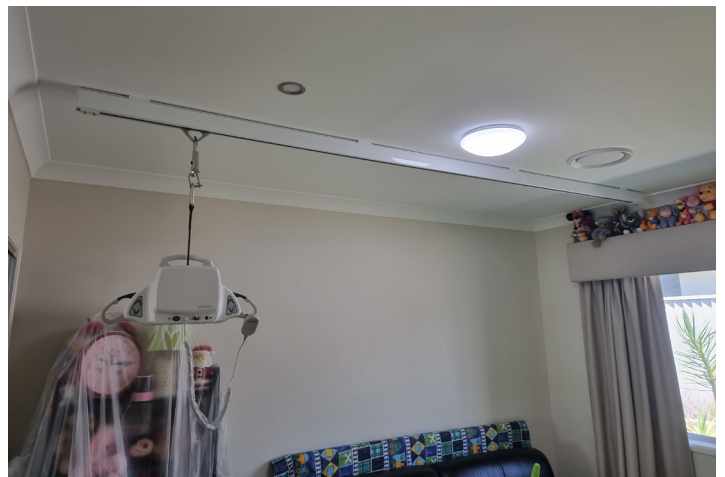
Straight track with portable motor
